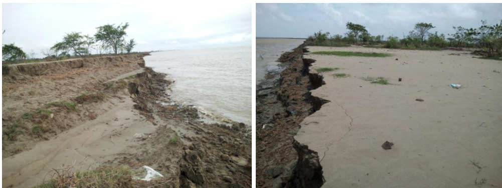
Plate 1 and 2. Eroded Bank of Sittaung River Mouth in Mamauk Village, Kawa Township
